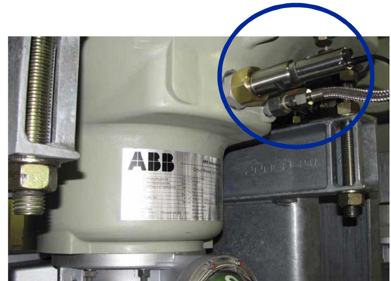
Humidity sensor on a GIS, Vaisala
